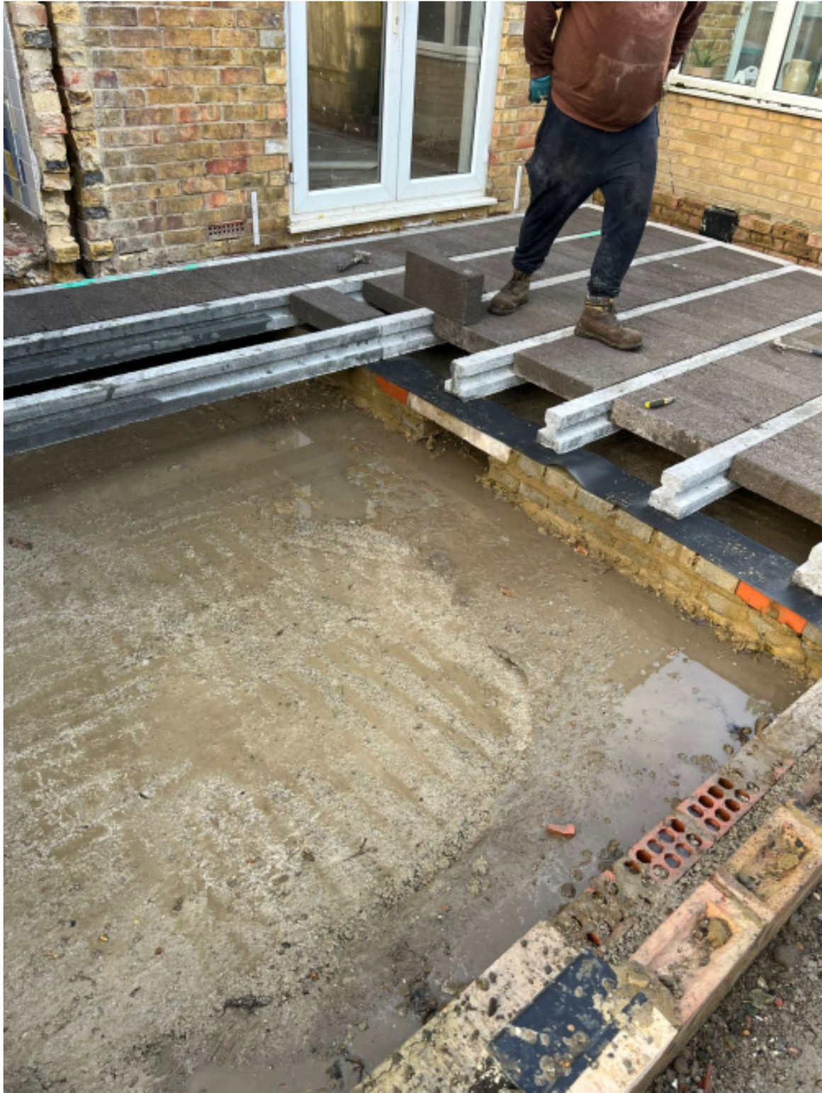
Fig 4 Surface water on concrete - Raining
